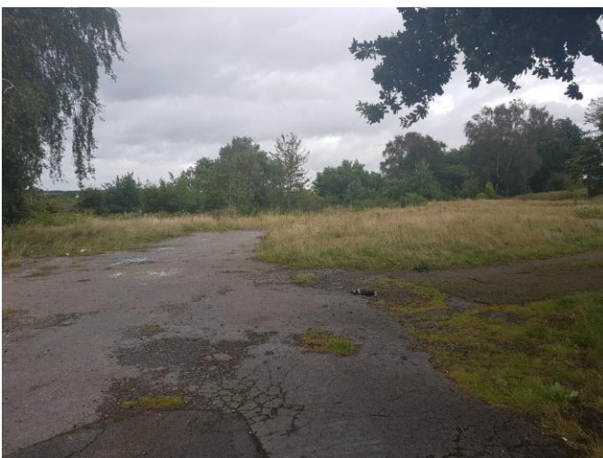
Poor internal access at St Matthew's on the Hill
