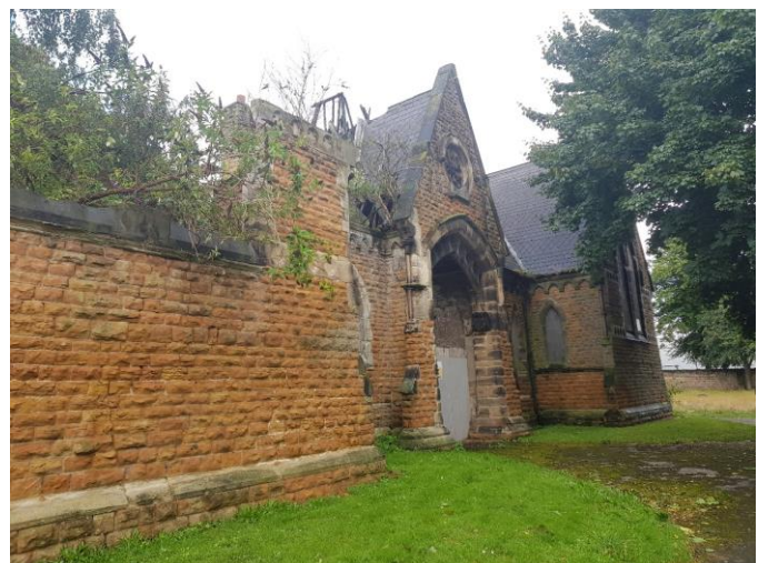
Chapel at Basford Cemetery in state of disrepair
